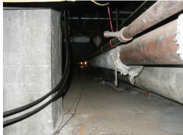
Friable Asbestos Pipe Insulation
